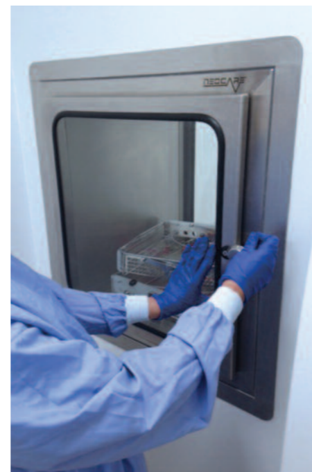
The endoscopy department has two ‘superb quality’, pass-through hatches with interlocked doors
